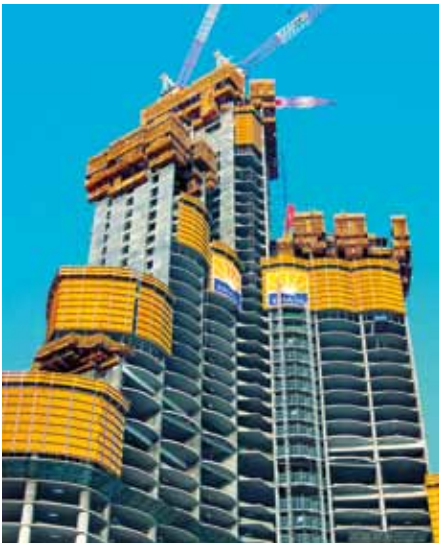
Sections for formwork have to have sharp edges. As a consequence there's no leakage of concrete and expensive re-grinding is avoided - as in the case of the construction of Burj Khalifa.
